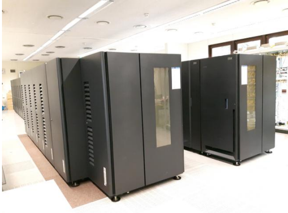
2 TS3500 Libraries OKD building
