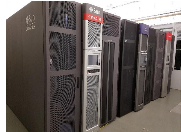
3 SL8500 Libraries SCC building
